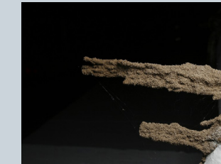
B - Termite mud tunnels/workings/galleries
