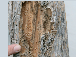
A - Termite damage in a timber fence
